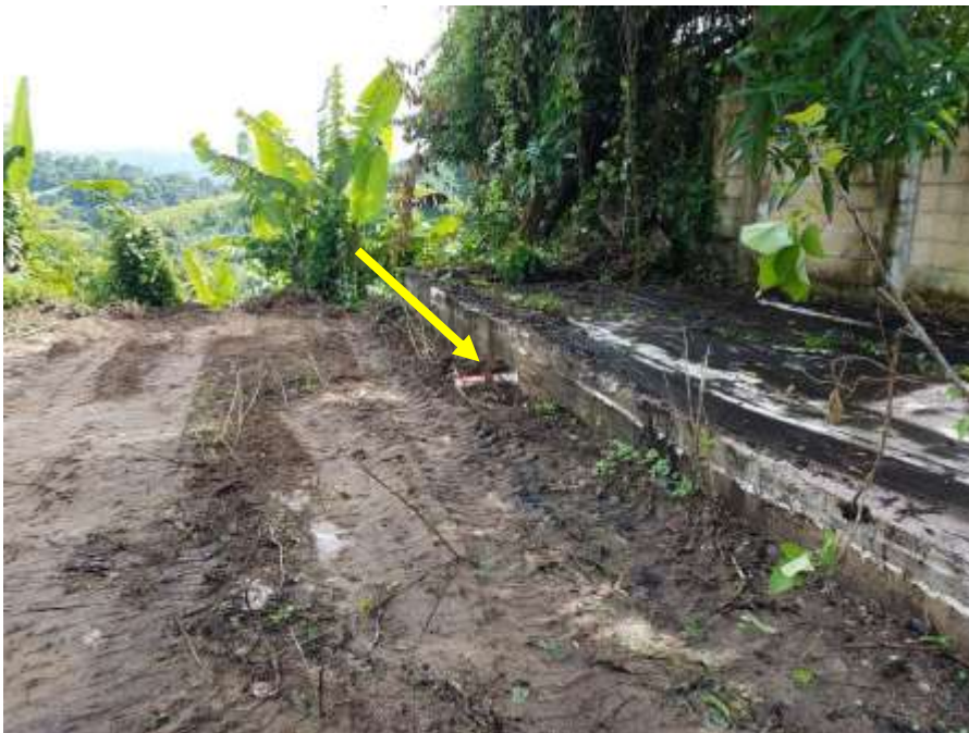
Photograph 16: PVC pipe discharging into ground surface.
