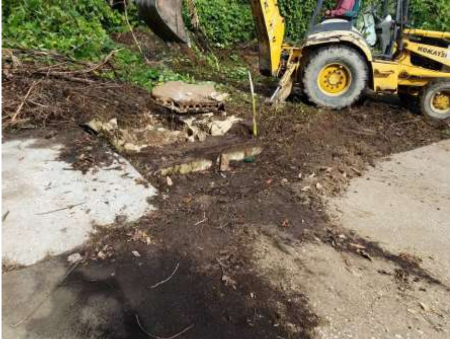
Photograph 15: Stained ground surface.
